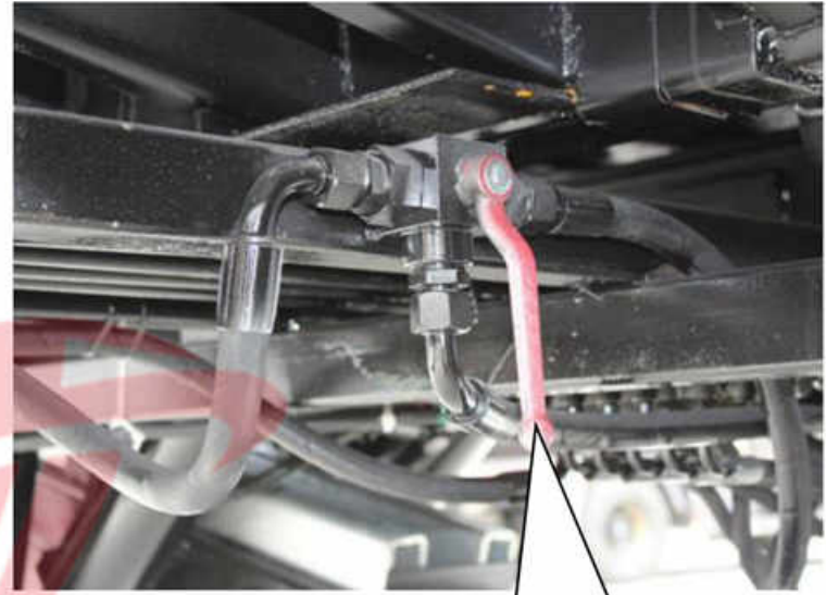
Figure 2: Red Switch vertical with platform
